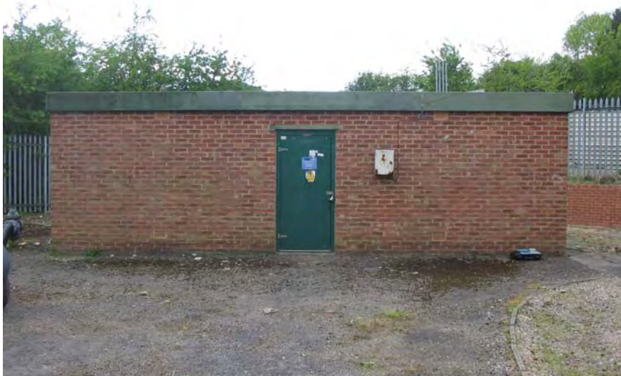
Figure 8.7 Brick built Kiosk housing a low-pressure twin stream district regulator. Four air vents can be seen; two at high level and two at low level. This pattern was repeated on the opposite wall
