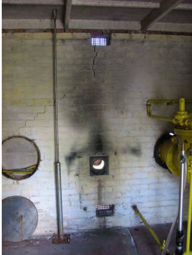
Figure 8.8 Photo taken from inside the building of the rear long side of the building. The circular opening has been created by the removal of equipment that once passed through the wall
