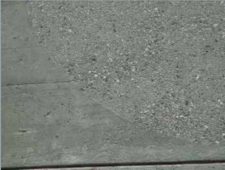
This photograph shows a concrete surface with the bocciardato texture next to the natural texture left from the formwork.
