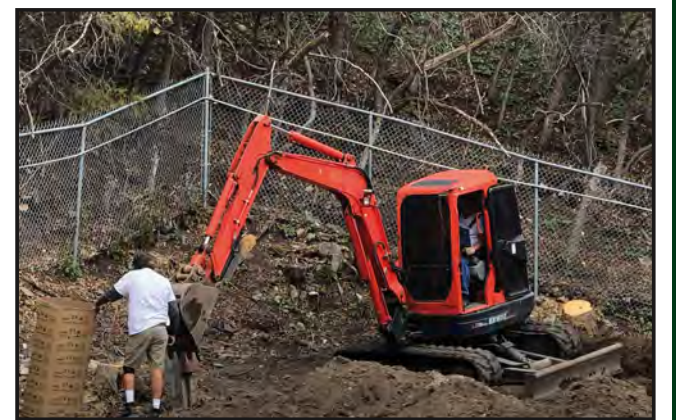
Tony Barker and Walt Shubert clearing space and digging footings in order to build yurt platforms at the Ophir Canyon Education Center.
