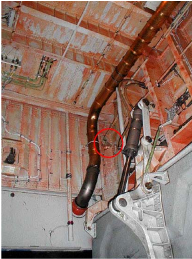
Figure 1 - View inside left main gear bay looking forward at the rear spar of the centre fuel tank. Purge door opening circled in red.
