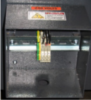
Power junction box without auto-transformer installed in the bandsaw.
