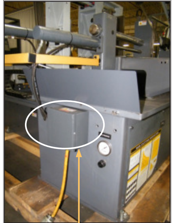
Power junction box
