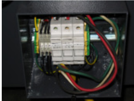
Power junction box with auto-transformer installed in the bandsaw.
