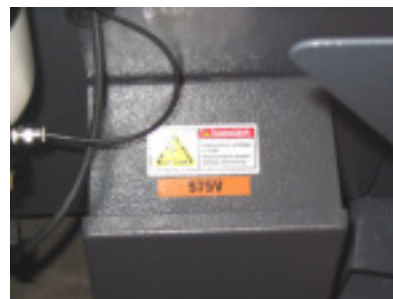
Power Junction Box.
