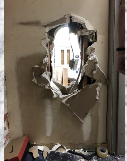
The narrow hole rendered through drywall between two studs gave looters access to Kicx's valuable merchandise locked in the basement of Pioneer Hall
