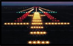
LED Runway Lighting and EFVS
