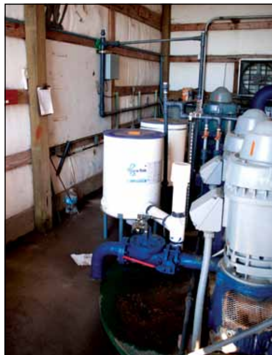
This nursery has a dedicated shed with chlorination treatment for disinfesting its irrigation water.
