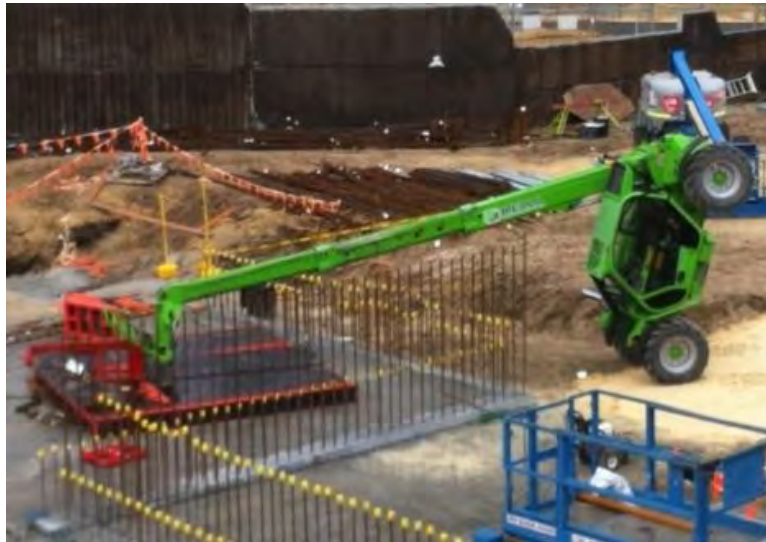
A telehandler was travelling with a large shutter suspended from the carriage when the machine tipped in a forward direction. The telehandler boom was at an unnecessarily high angle and the load was outside the height/radius permitted by the load chart.
