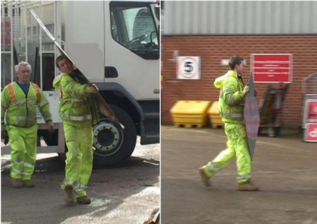
Figure 9. TMO carrying rigid wicket sign (left) and 'works traffic only' sign (right)
