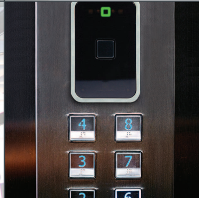
Elevator Access Control
