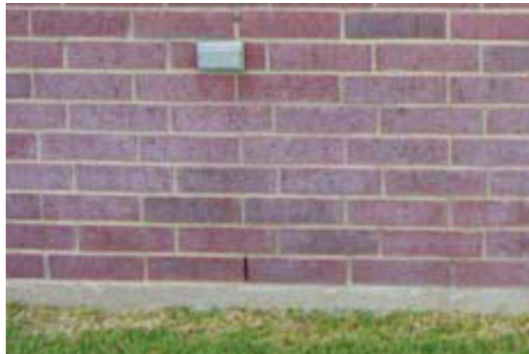
Figure 5.8: Stains from Running Water
