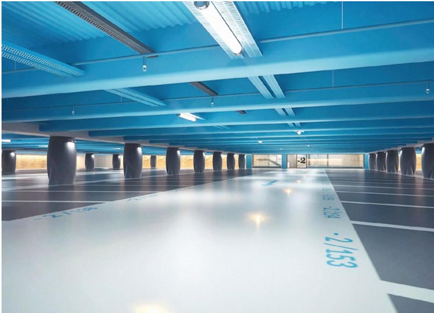
34 Blox, Copenhagen (Danemark), OMA. Luminaires: Benson Parking, Lyon, Tomasini Design. Luminaires: Géricault
