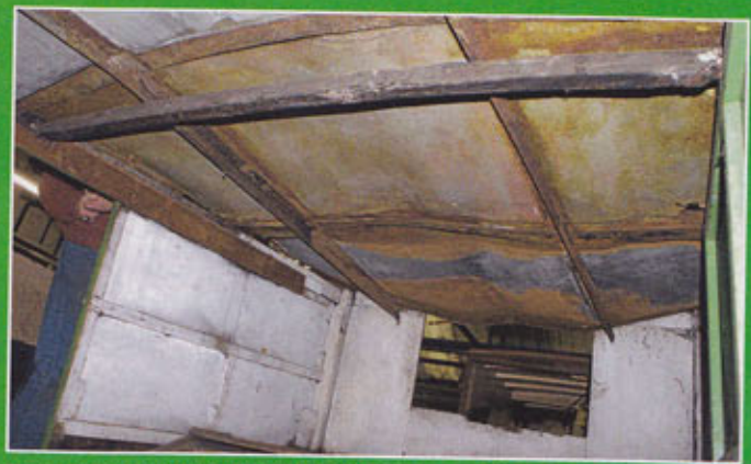
The roof was simply a collection of metal patches over the one remaining roof stick and added metal angle iron.
