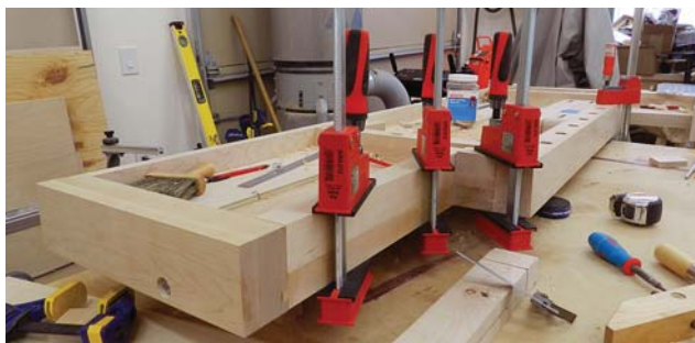
Tail vise filler. I used the offcut from the vise recess to block in the edge of that recess with 2 1/4"-thick pieces in an L shape – that beefs up the opening to the same thickness as the vise to come. I glued it and pocket screwed it (just in case the glue ever fails).
