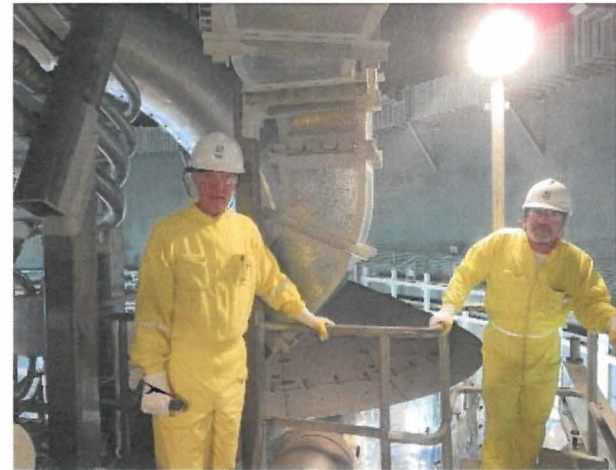
NRC Staff at top of the Sanmen Unit 2 steam generator
