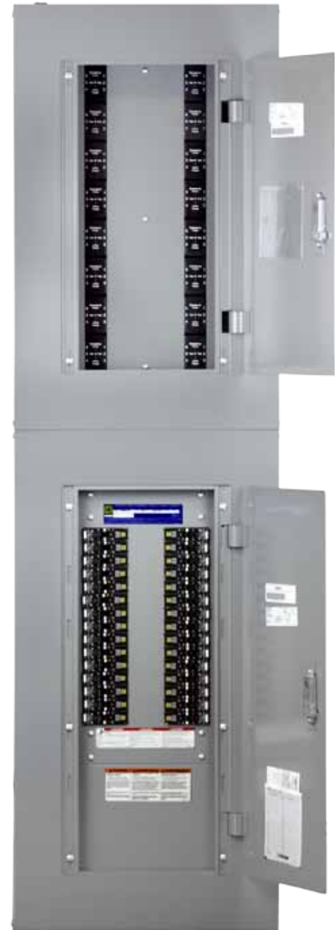
Emergency Lighting Control Panelboard
