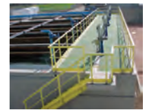
Gangway in water treatment.
