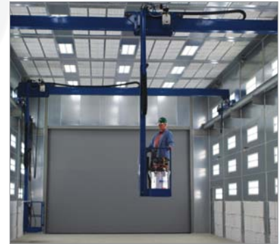
Overhead Lift System
