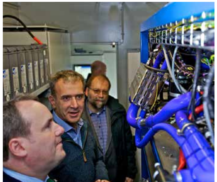
Paul Wheelhouse MSP at the 'Surf n Turf' hydrogen fuel cell training compound, Kirkwall, Orkney. (Credit: Colin Keldie)
