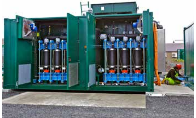
Surf 'n' Turf hydrogen electrolyser, Orkney (Credit: Colin Keldie)
