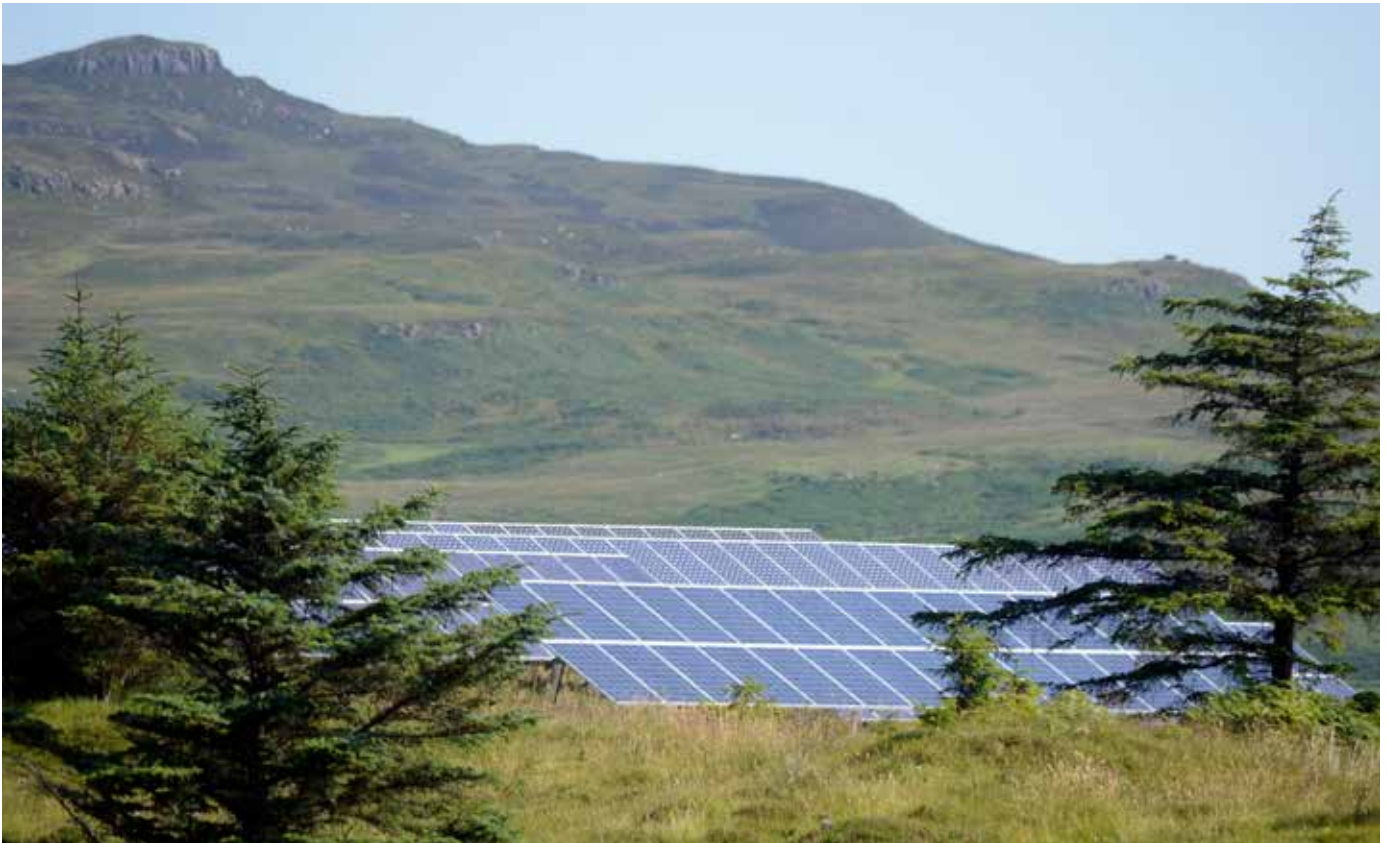
Solar PV array on the Isle of Eigg, Inner Hebrides; part of a community owned renewable electricity system on the island. (Credit: Highlands and Islands Enterprise)
