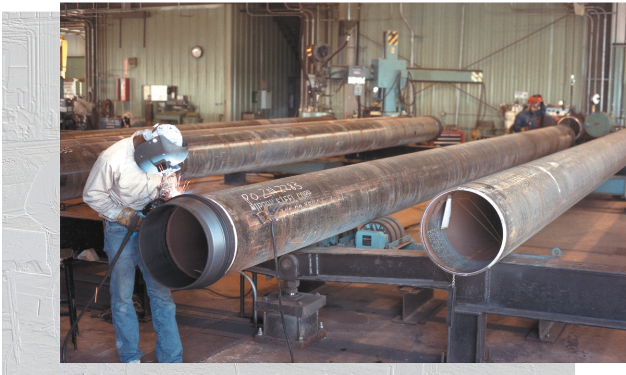
At Vetco Gray, our welders are trained and certified to ensure the integrity of the materials.
