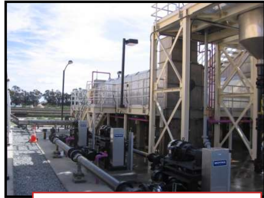
Monterey CA, WWTP, Screw Press
