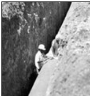
These workers are not protected from a cave in, nor do they have any apparent safe access or egress from the trench.
