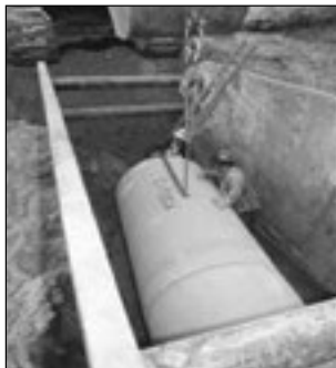
These workers are protected from a cave in and have safe access and egress from the trench.
