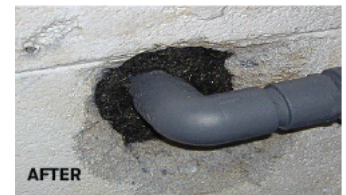
Stainless steel mesh fabric is the most effective material to keep rodents from entering through building holes and penetrations.
