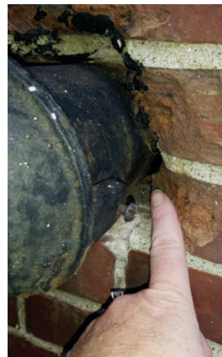
Jody Gangloff-Kaufmann, NY State IPM Program Inspect areas where pipes and wires enter buildings to determine whether pests can enter around them.
