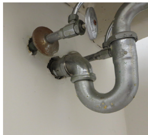
MATT FRYE Openings around utility lines often provide access to buildings and wall voids.
