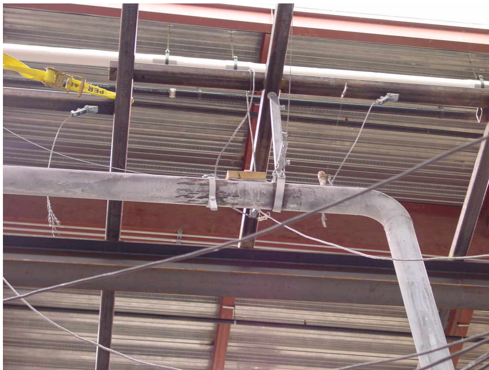
Figure 10. Brace #B11 Failure
