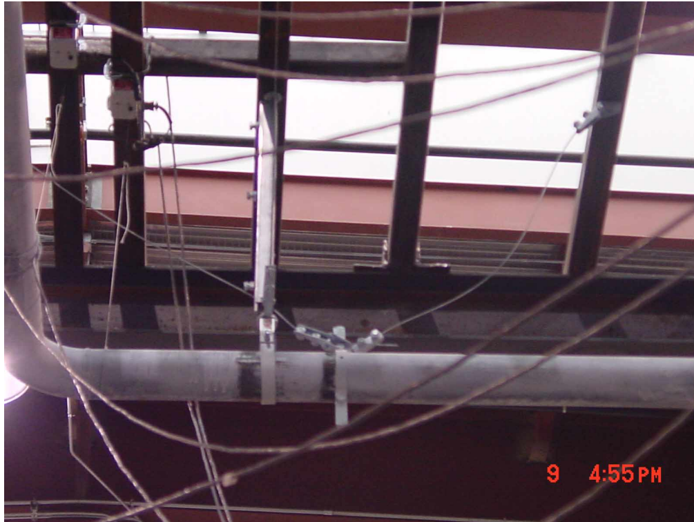
Figure 12. Permanent Displacement of Brace #B7
