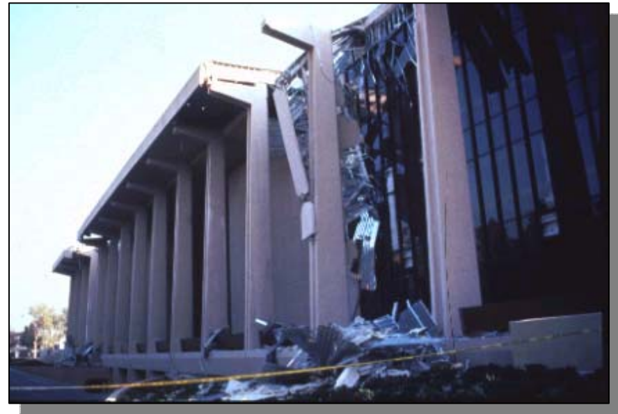
Exterior damage to the back (north side) of Oviatt Library during Northridge Earthquake (attributed to pounding).
