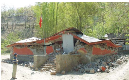
(a) Poor cement mortar in the elementary school building (Emre et al, 2003)
