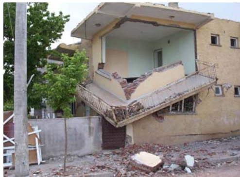
Figure 15 A failure occurred around the balcony of a masonry building during Bingöl Earthquake
