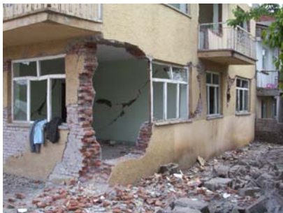
(a) Damaged during Bingöl Earthquake
