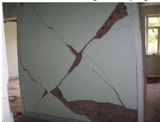
Figure 9 Typical X cracks occurred in the load-bearing inner walls during Bingöl Earthquake
