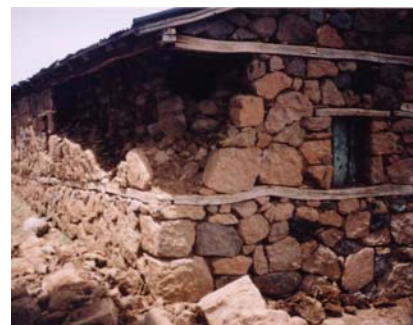
(b) Poor mud mortar
