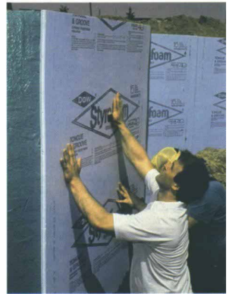
Thwarting condensation. An insulating board provides protection from backfill and helps eliminate interior condensation. Photo courtesy Dow Chemical Company.
