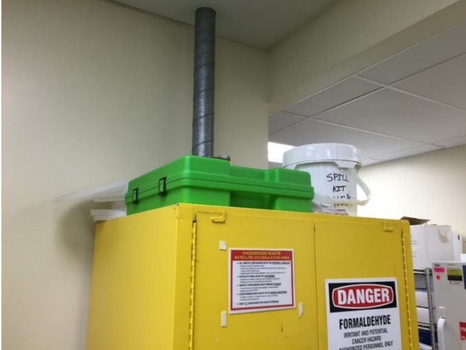
Figure 34 Ventilated Flammable Gas Cabinets
