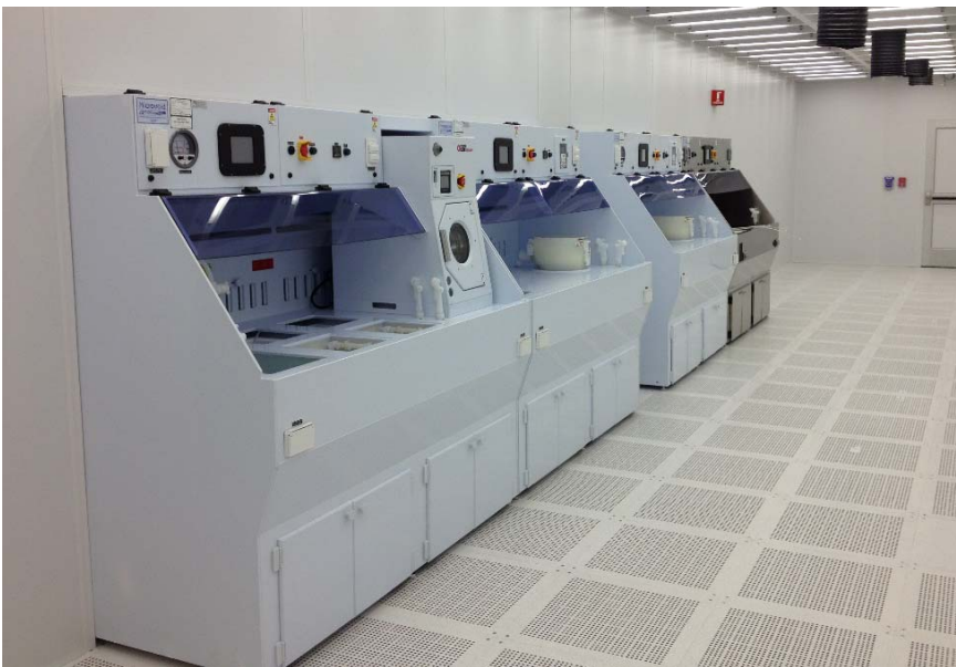
Figure 33 Wet Process Workstations
