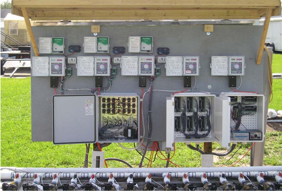
Figure 2-8. Control board showing timers, soil moisture sensor-controllers, solenoid valves wiring, and flowmeters-datalogger (details are shown in the next Figures).
