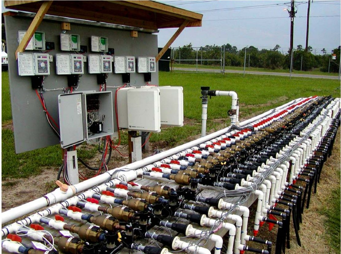
Figure 2-6. General view of the irrigation controls used in this study.
