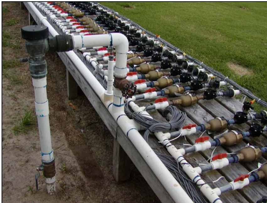
Figure 2-7. Pipes, flowmeters, valves, and wirings for this study.
