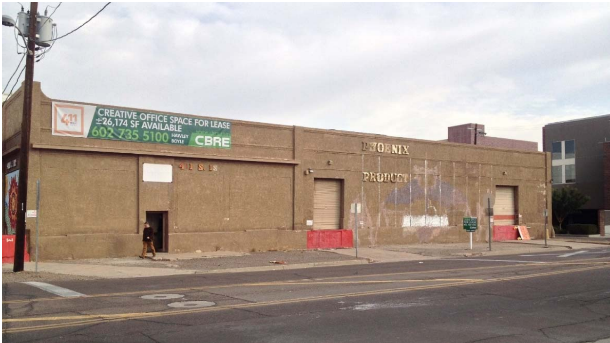
Photo 1. View of west façade of 411 South 1 st Street depicting infilled windows and stucco sheathing, prior to rehabilitation, facing southeast (2016).
