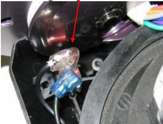
Check Voltage at top terminal
