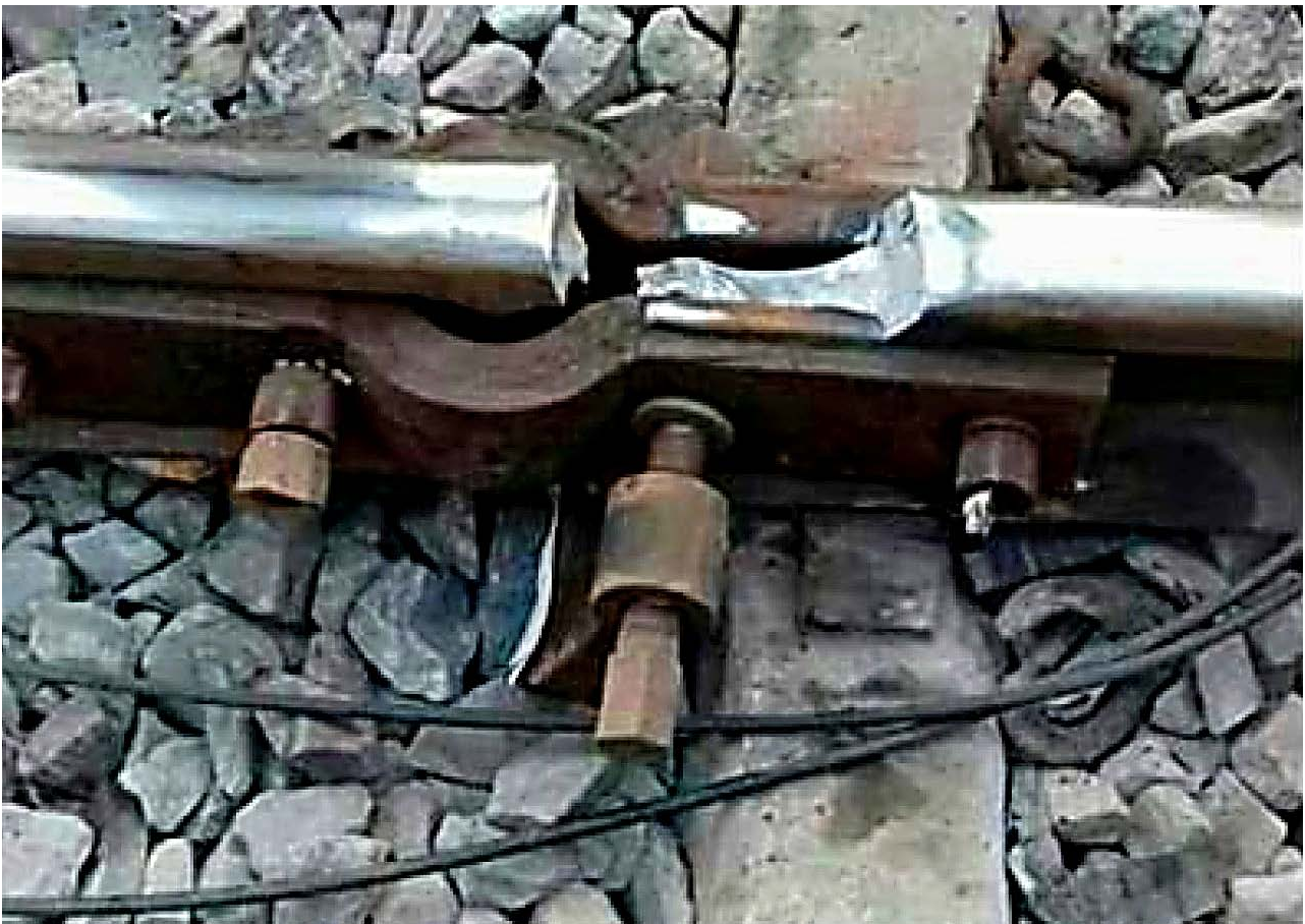
Rail/Weld Fracture prone Track ; Kalyan 2016
