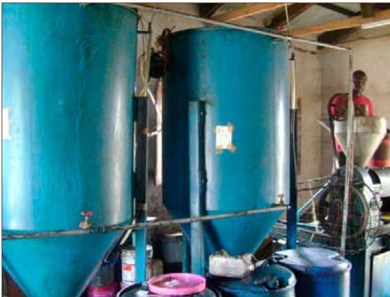
Fig. 4.9. Oil storage tanks (Photo from L. Gedi)
