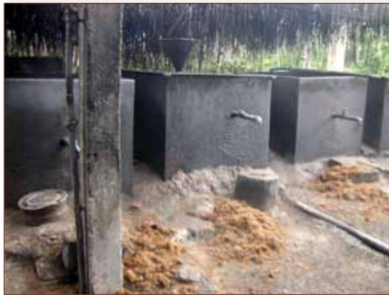
Fig. 4.7a and b. Oil clarifiers (Photo from J. Hounhouigan)
