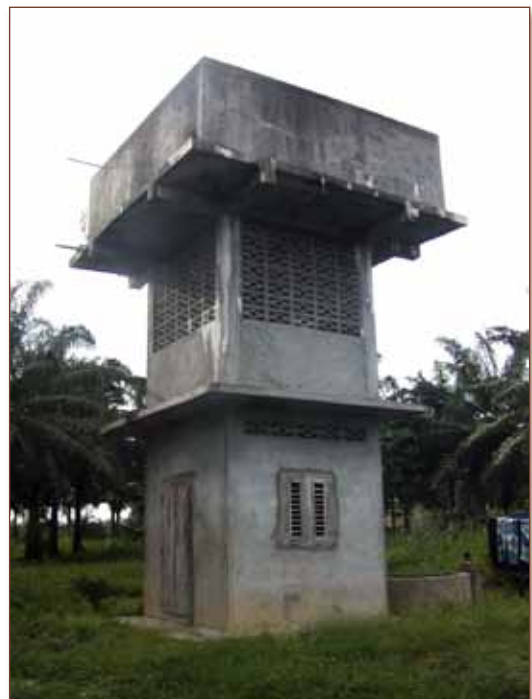
Fig. 3.2. Example of a water tower constructed in a palm plantation to supply a palm oil processing unit (Photo from J. Hounhouigan)
