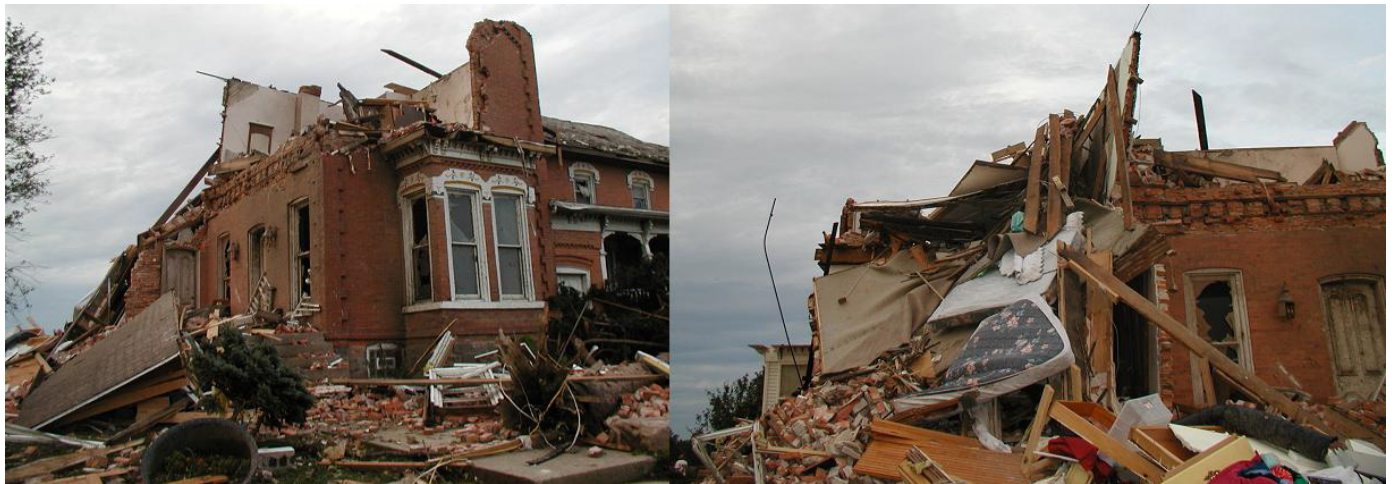
This brick building was heavily damaged by the tornado that brought winds of well over 100 mph.
