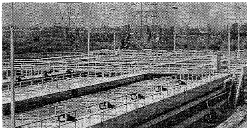
Figure 5-1. Sewer line root control pesticide applications can have serious impacts on wastewater treatment plants unless proper planning takes place before application.
