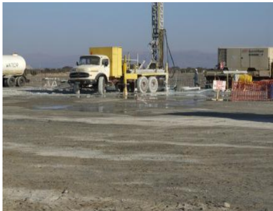
Picture 4 (above) Sub Contractor in progress with the drilling of one 165 mm X 170 metre hole.
