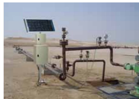
The Sensornet Oryx DTS has been designed for remote monitoring in harsh environments
