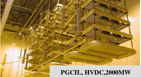
PGCIL, HVDC, 2000MW
