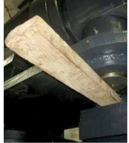
A plank supports emergency-closure valve pins in the Kajaki Dam Irrigation Tunnel. (SIGAR photo)
