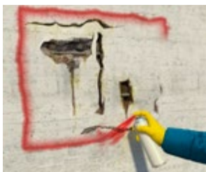
Identify and assess damage.
