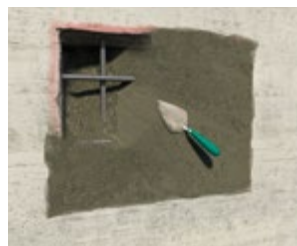
Press Sika MonoTop®-412 N into the repair area using a suitable hand tool.
