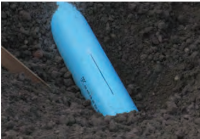
Water pipe cut.
