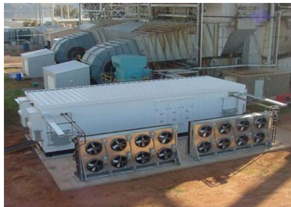
Example of installation with W32 option: there are 2 WC drives in the building
