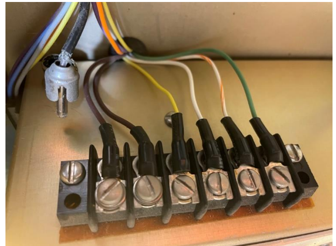
The wire terminal block on the RF Deck. These wires had to be disconnected.
