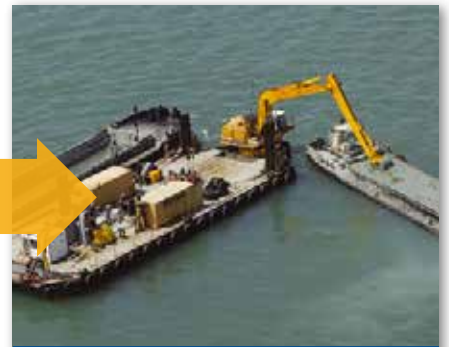
3D Submersible Machine Control
