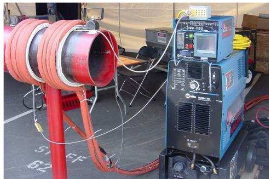
Figure 9.64: Induction heating: Primary insulated winding induces current into lossy iron pipe (secondary).
