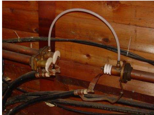
Figure 14.52: Flexible coaxial cables connected to rigid lines.
