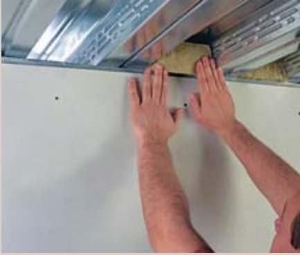
Mineral Wool is placed in the fluted metal deck after the drywall is installed.
