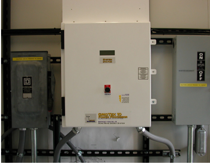
Figure 2. Gridtek inverter and disconnects
