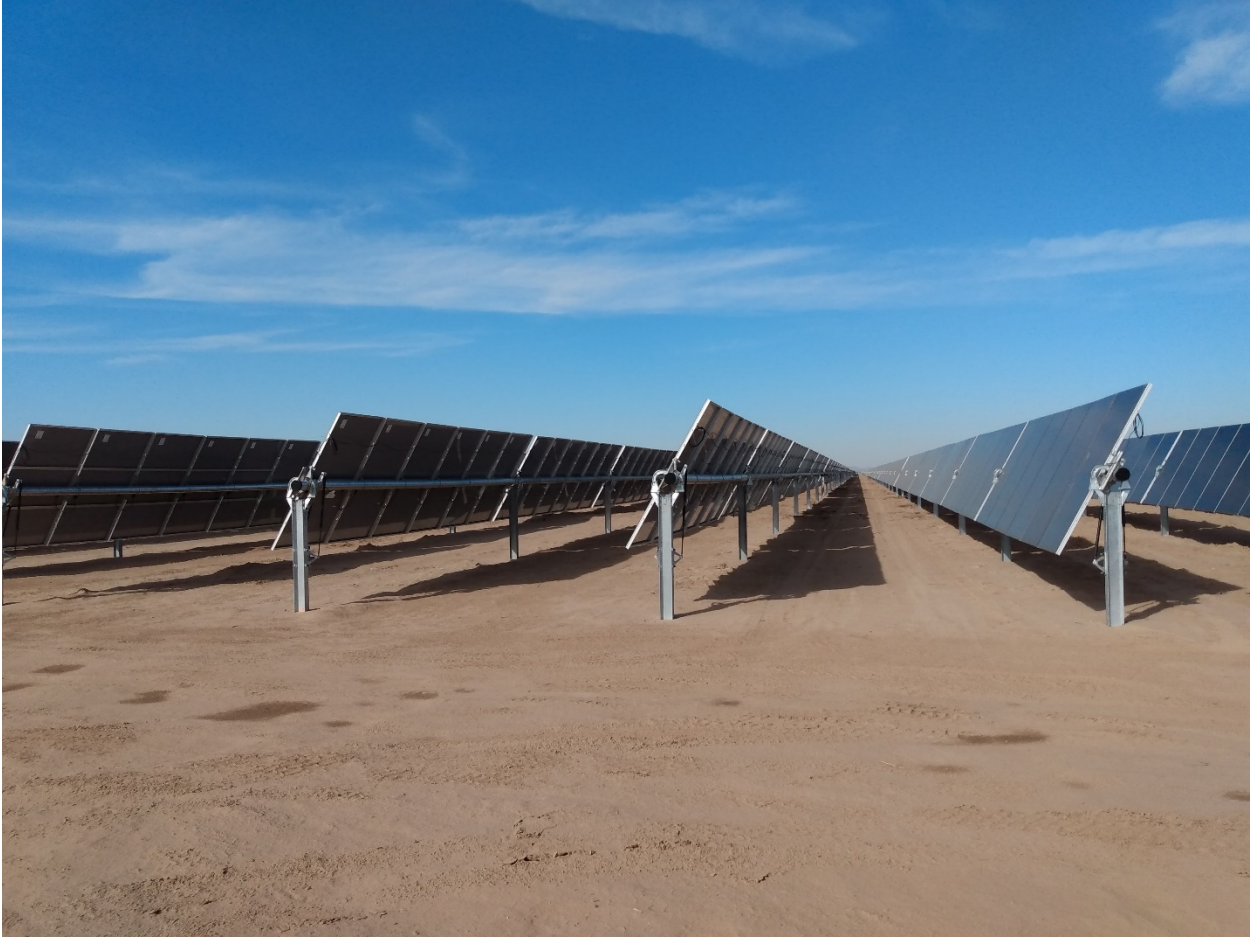
Figure 2 – Single-axis Tracker Panel Strings
