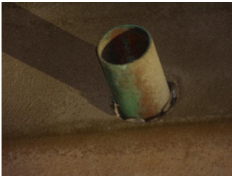
Image 6 - Unsealed vent / overflow
