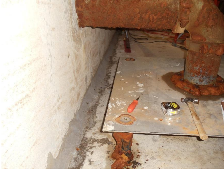
Image 3 Fire Pump Inlet
