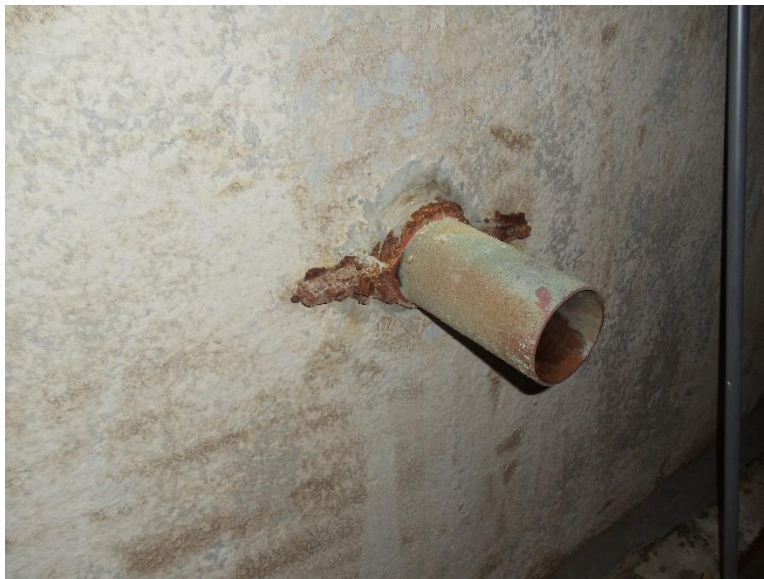
Image 2 - Recirculation intake penetration
